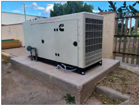
A. New emergency power generator for Campus Server and Communications Room
